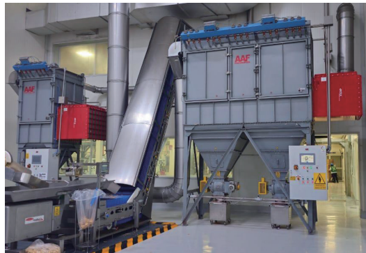
WONDAIR™ at customer's plant
