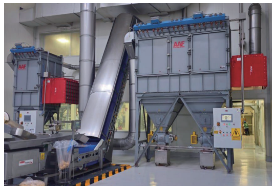
WONDAIR™ at customer's plant
