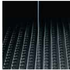
Scan test showing leak indicated by a smoke trail.
